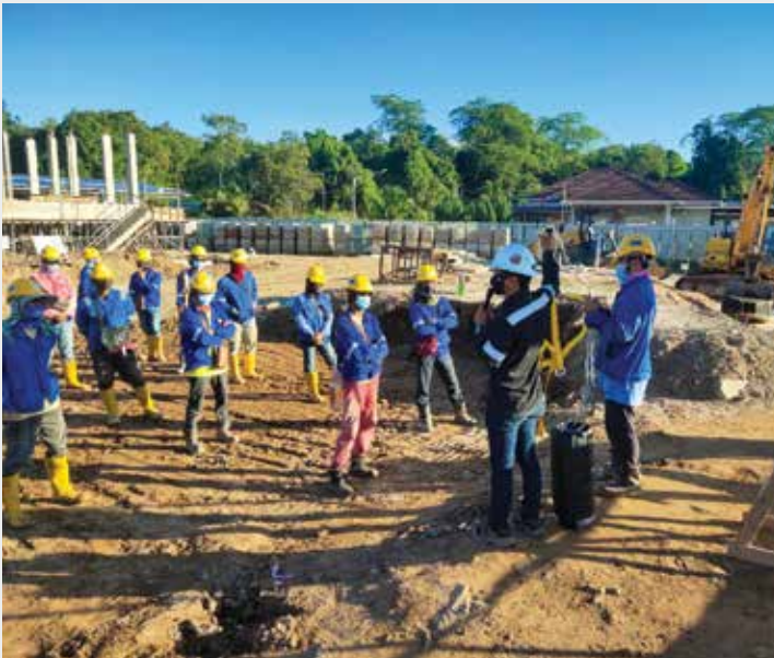
Ⓞ Awareness Training on Safe Use of safety body harness at Limbang Town 275/33/11kV substation project.
